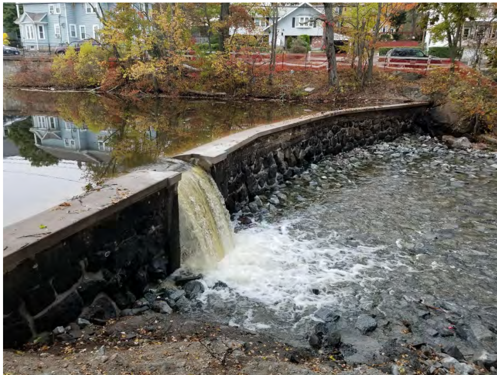
Photo No. 20 – Photo taken in November 2017 at the completion of rehabilitation construction.
