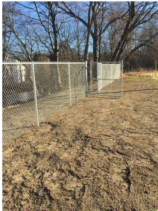
Photo No. 10 – Chain link fence installed between Condon Park and right bank.
