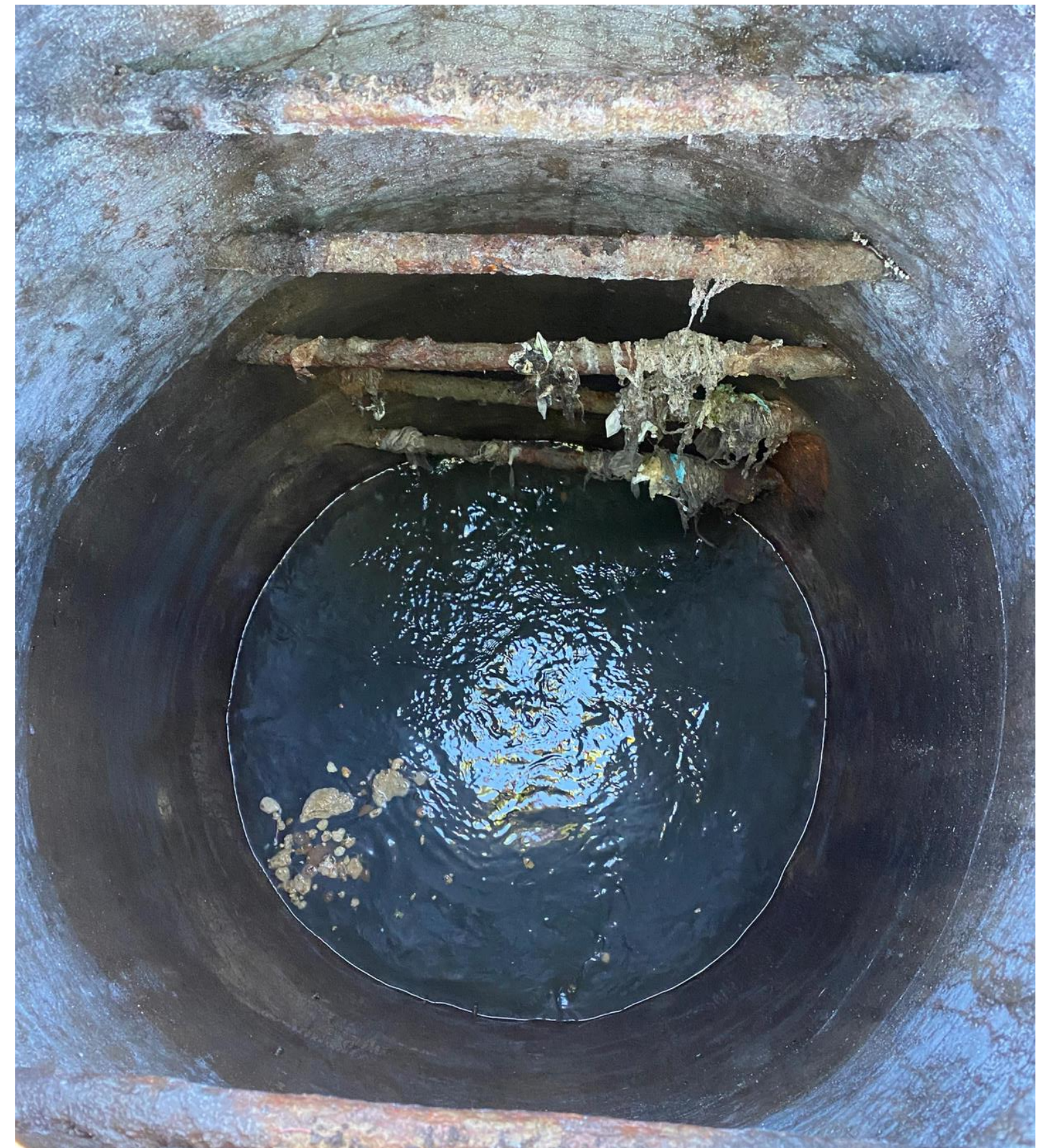
Surcharged Sewer Manhole
