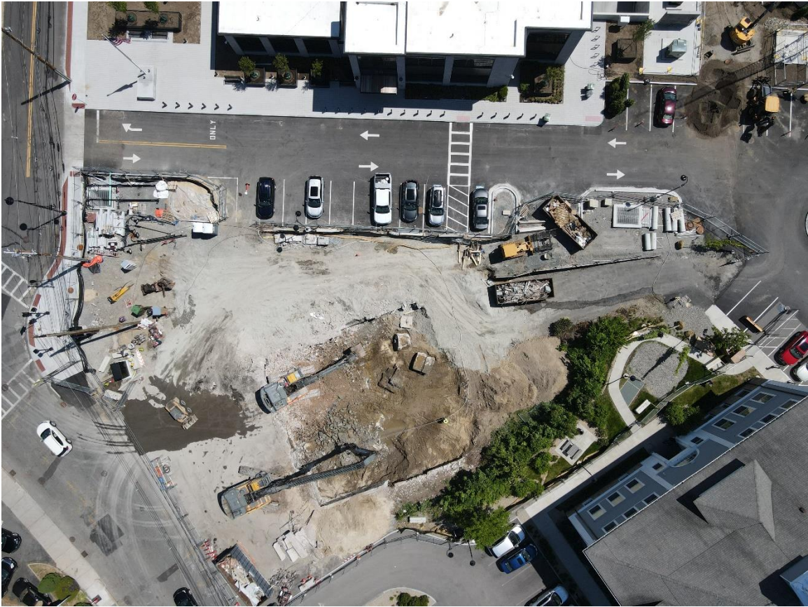
Caption: Overhead view of the site of the former Fire Station Building taken via drone on Friday, May 26, 2023. Upon completion, this area will include parking and landscaping to complete the Municipal Campus of Town Hall and the new Public Safety Building. Work is expected to be completed in Fall 2023.
