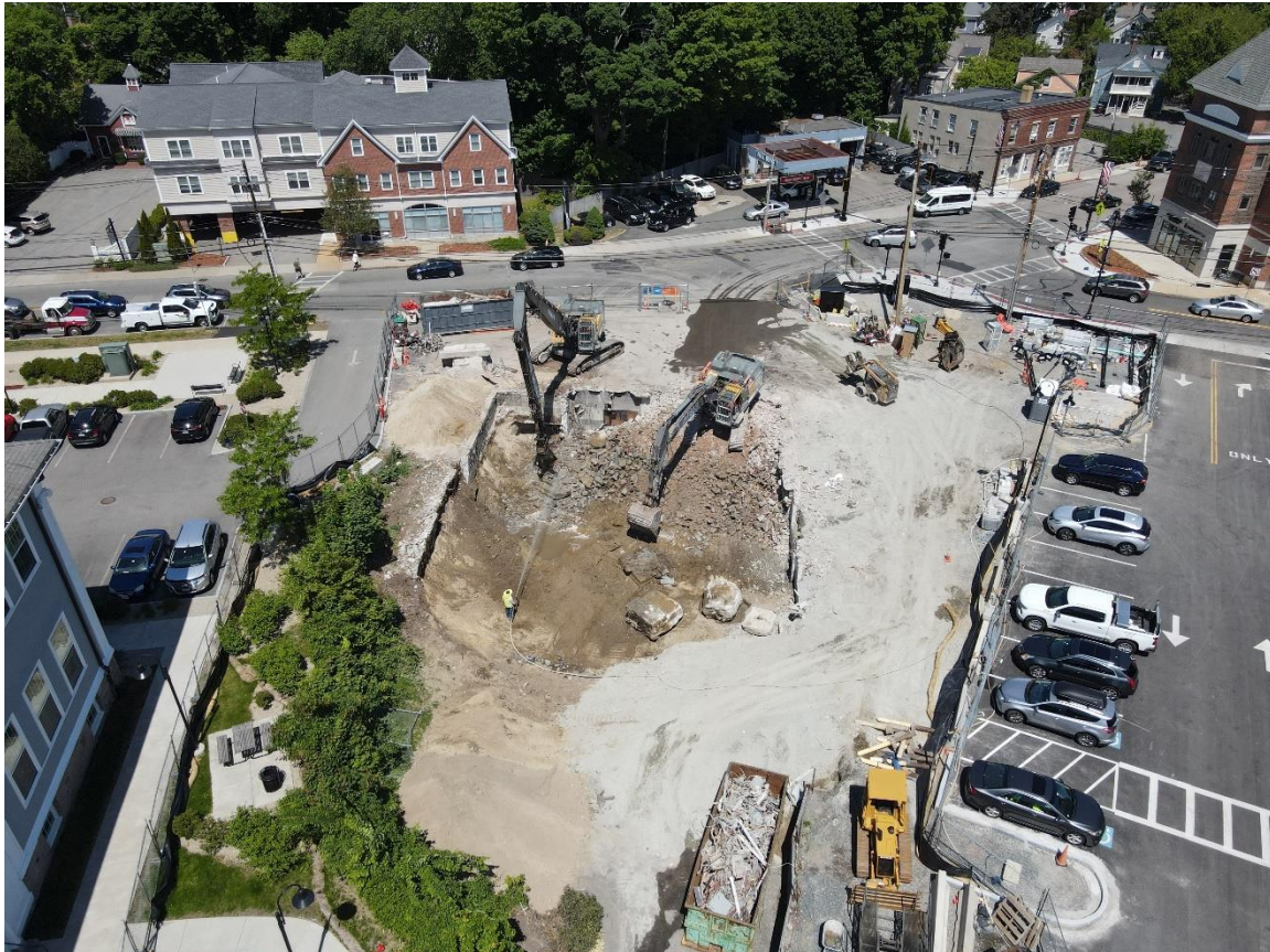
Caption: Aerial photo of excavators clearing materials from the site of the Former Fire Station building following demolition, taken Friday, May 26, 2023 via drone.
