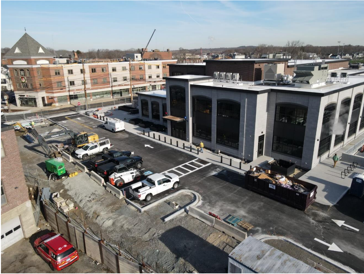
Caption: Photo of the active construction site facing the south side of the building at the new public entrance, taken on Wednesday, December 21, 2022. Crews have completed the parking lot striping to show the two lanes of travel and visitor parking spaces adjacent to the lined crosswalk.
