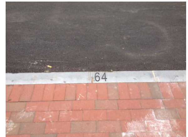
Stall (space) number etched into the granite curbing.
