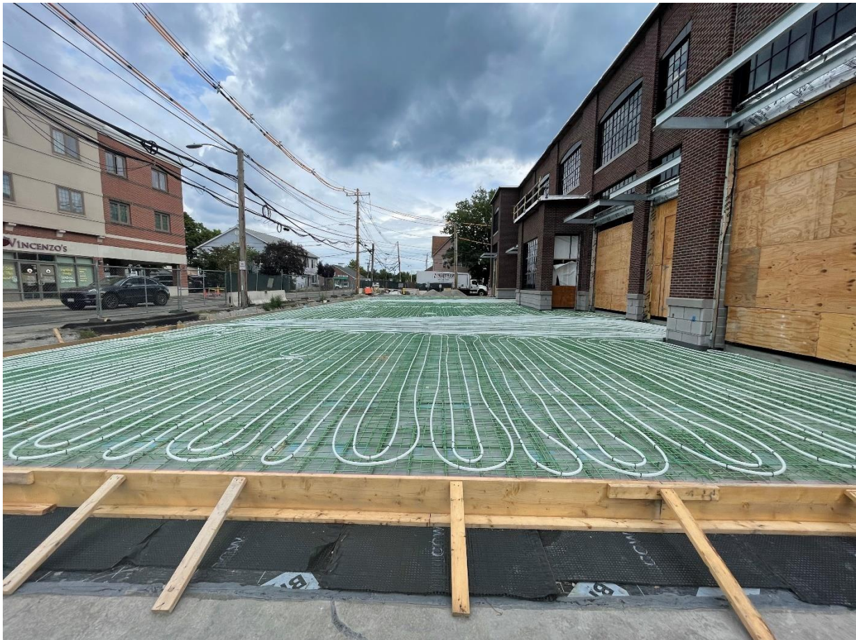
Caption: Photo of the newly installed snow melt system located outside the north side of the building in front of Fire Station, taken on Wednesday, August 17, 2022.
