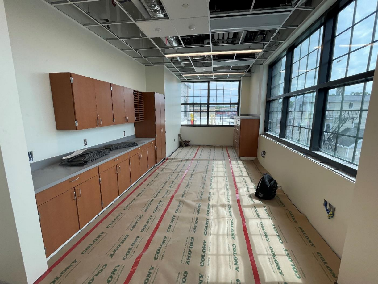
Caption: Photo of a workspace for Police Detectives under construction, taken on Wednesday, August 17, 2022.
