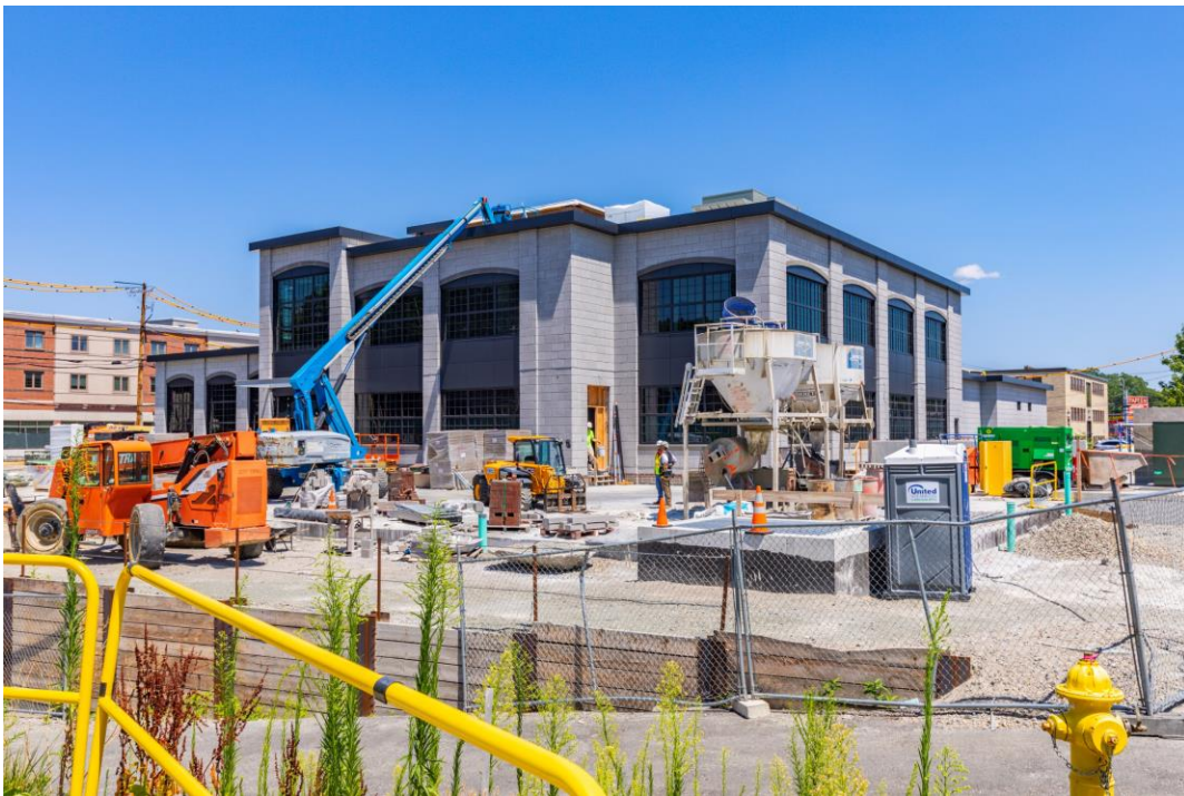
Caption: Photo of the active construction site taken from the north side of Town Hall on July 22, 2022.
