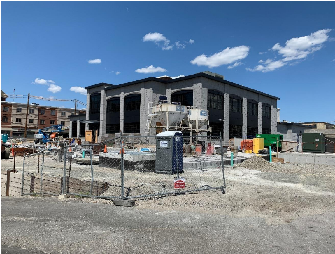
Caption: Photo of the active construction site taken from the north side of Town Hall on July 15, 2022.
