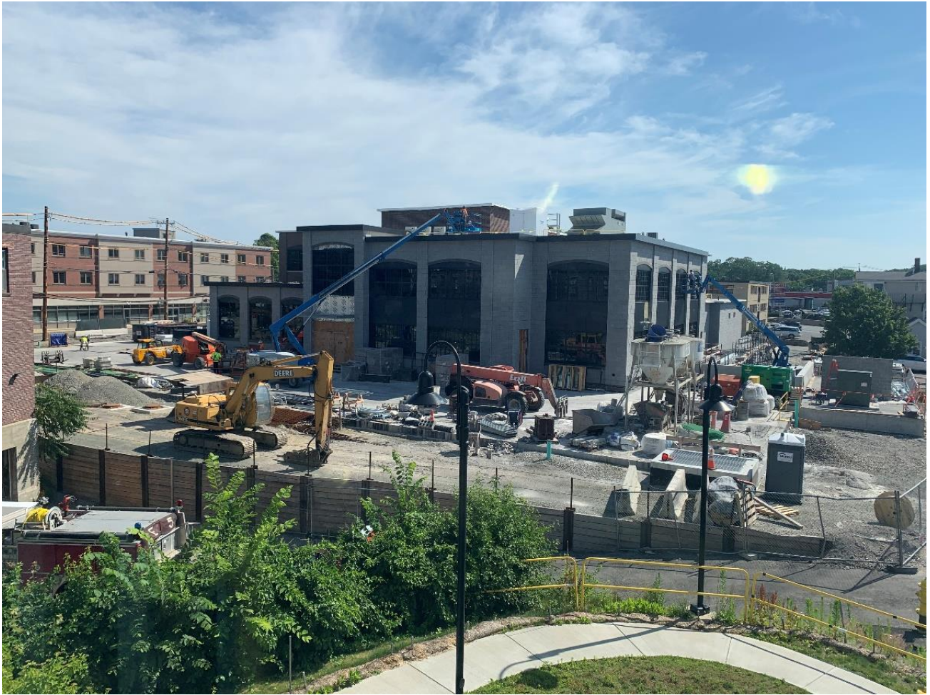
Caption: Photo of the active construction site taken from the north side of Town Hall on July 1, 2022.
