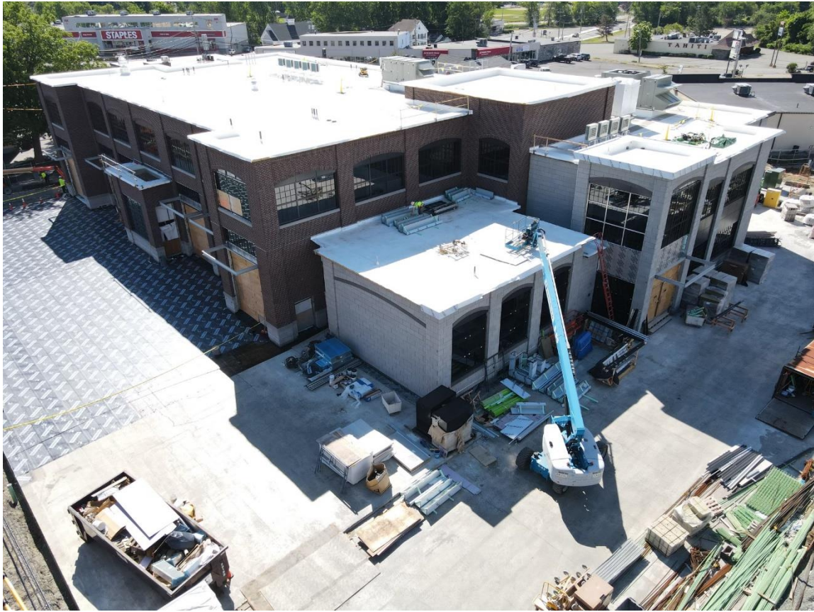
Caption: Photo of the active construction site on Tuesday, June 14, 2022 via drone facing east. The exterior stone and brick masonry work has been completed and contractors are shown to the center right of the photo loading materials to the roof via small crane and lift.
