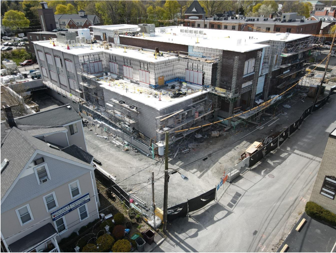
Caption: Photo of the active construction site taken via drone facing the north corner of the building on Thursday, April 28, 2022.
