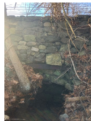
'Failing' Dry Laid Stone
