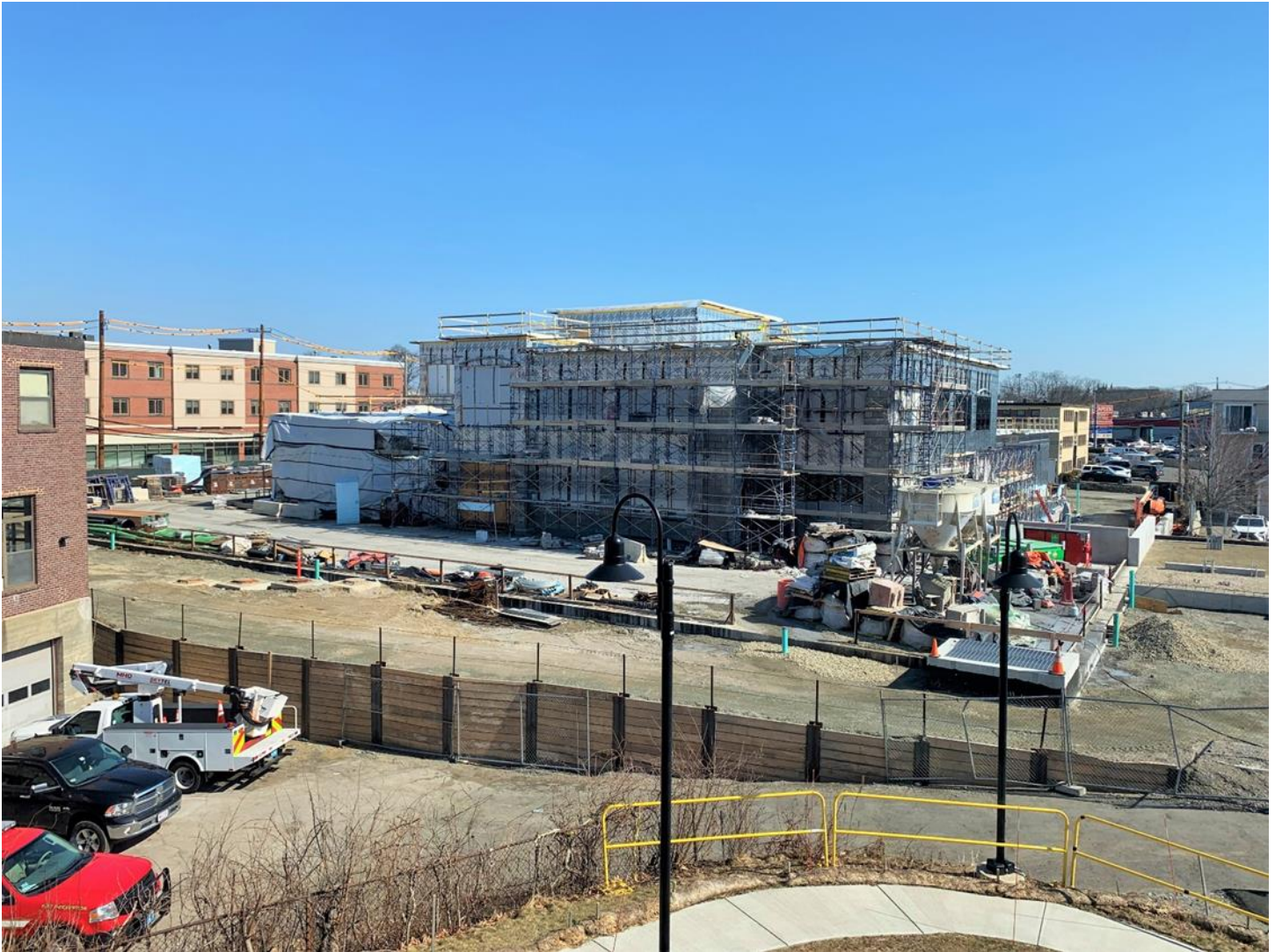
Caption: Photo of the active construction site, taken from the north side of Town Hall on Friday, March 18, 2022.
