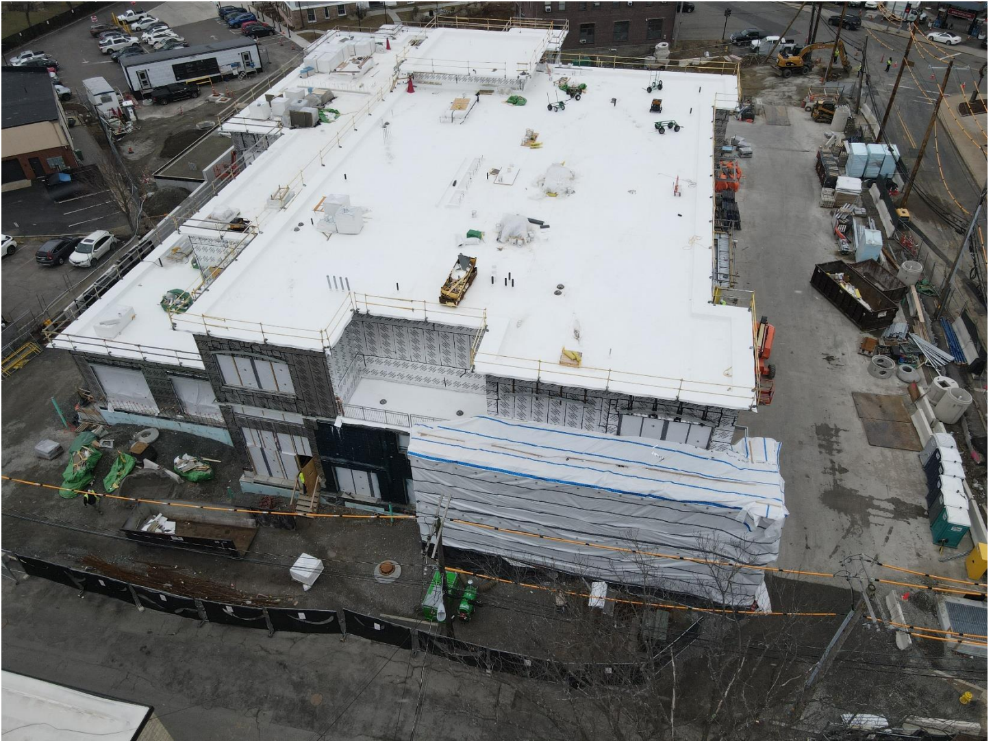
Caption: Photo of the active construction site, using a drone on Wednesday, March 9, 2022. Crews are still installing the exterior stone veneer, Shouldice, on the west and north sides of the building. The white plastic sheeting on the exterior of the building helps to protect the stone veneer during installation and while the mortar cures.
