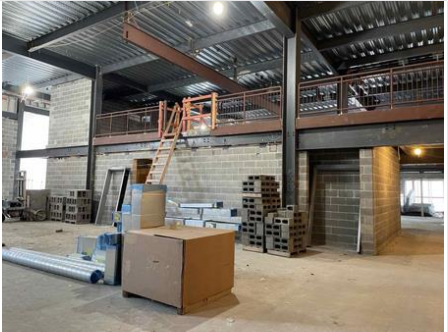
Apparatus Bay Hoist Beam - Mezzanine Guardrail System
