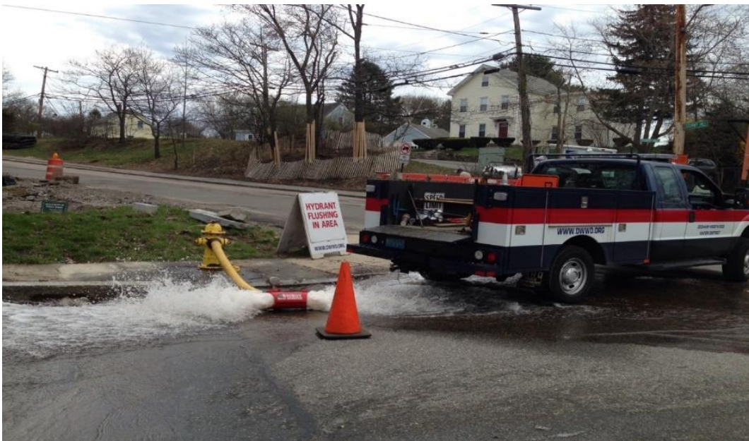
Caption: DWWD truck flushing hydrant along roadway as part of regular flushing program
