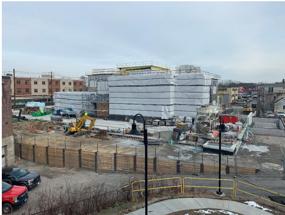
Caption: Photo of the active construction site taken from the north entrance to Town Hall on Friday, January 28, 2022.
