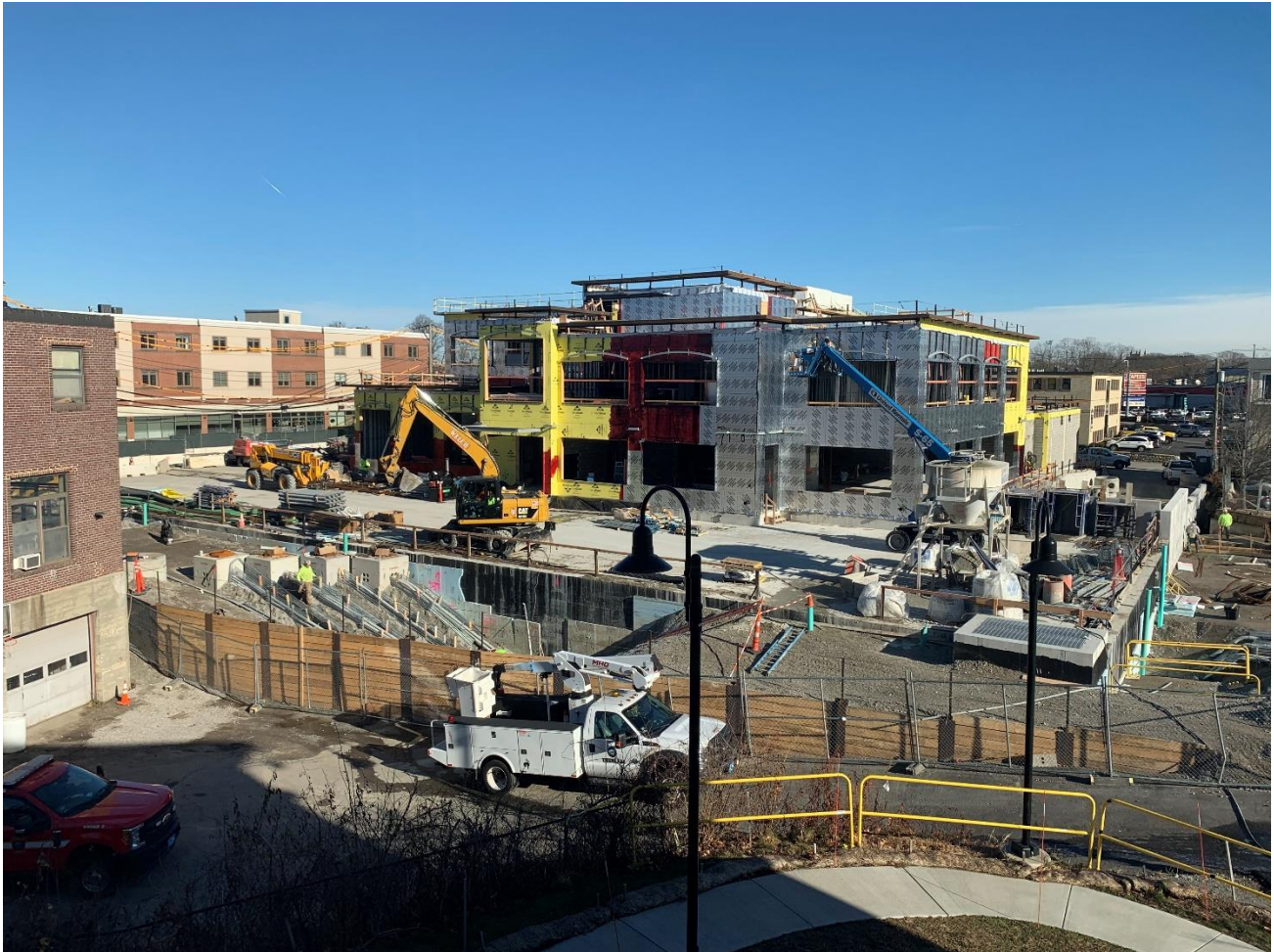
Caption: Photo of the active construction on Monday, December 20, 2021 taken from the north side of Town Hall.
