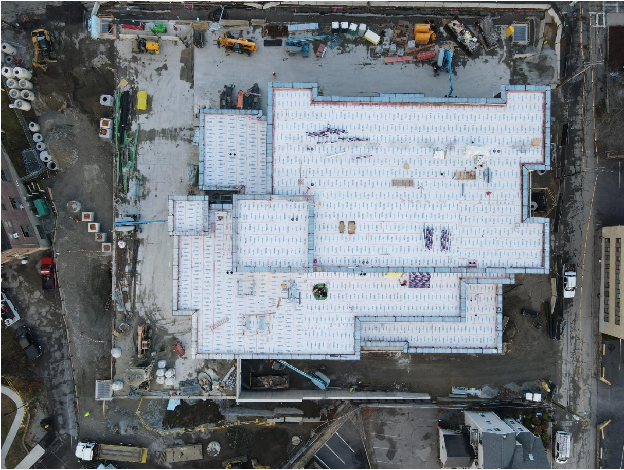
Caption: Aerial photo of the active construction site taken using a drone on Friday, December 3, 2021. The white material shown on the roof the building is the air vapor barrier. As of Friday, December 3, crews had successfully completed the installation of air vapor barriers on the roof.
