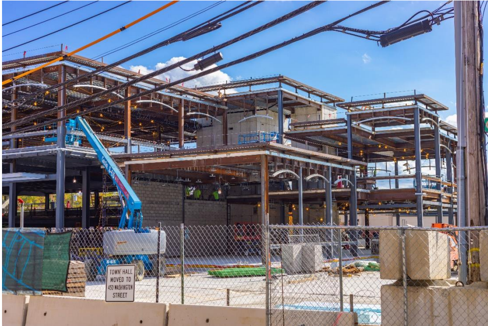
Caption: Photo of active construction site taken from Bryant Street, taken on Friday, October 22, 2021.
