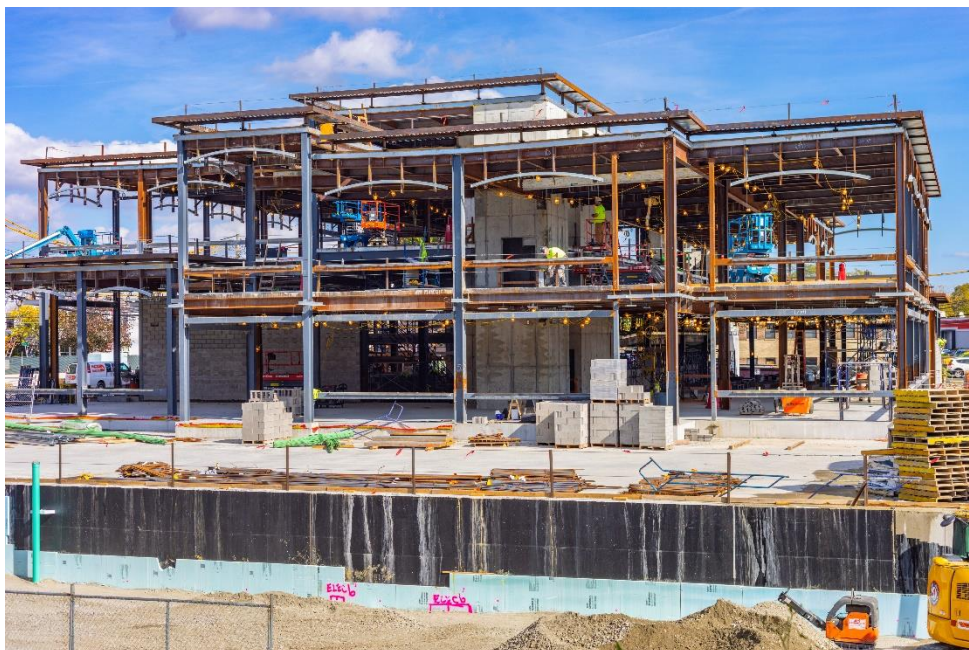
Caption: Photo of active construction site taken from the north side of Town Hall on Friday, October 22, 2021.
