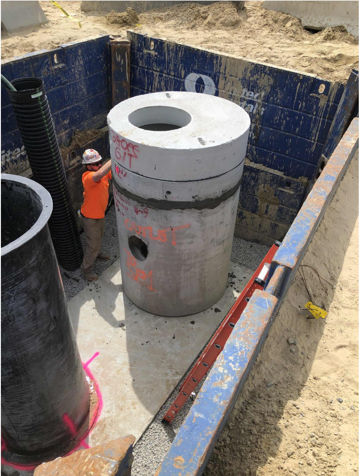
Sub-slab utility tanks
