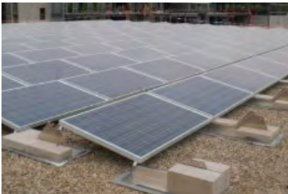
Solar panels as part of the Dedham Municipal Solar Project are helping the Town to source more of its energy from renewables.
